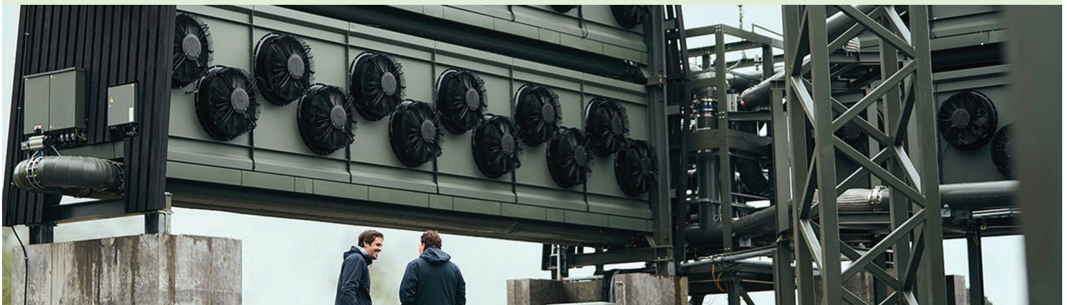
The Climeworks Orca direct air capture facility in Hellisheidi, Iceland launched September of 2021 with a capture capacity of 4,000 tons making it the largest operational direct air capture project to date. Credit: Climeworks.
