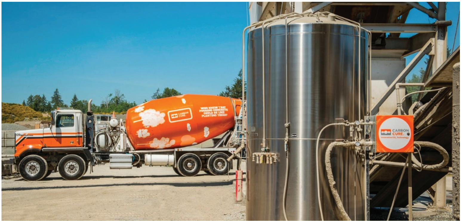
Canadian company CarbonCure injects captured CO 2 into fresh concrete where it undergoes a mineralization process and remains permanently embedded, thus reducing the overall carbon footprint of the product. In April 2021 CarbonCure won the NRG COSIA Carbon XPRIZE, a global competition where competitors develop breakthrough technologies to convert CO 2 into usable products. Credit: Carbon Cure Low Carbon Concrete.
